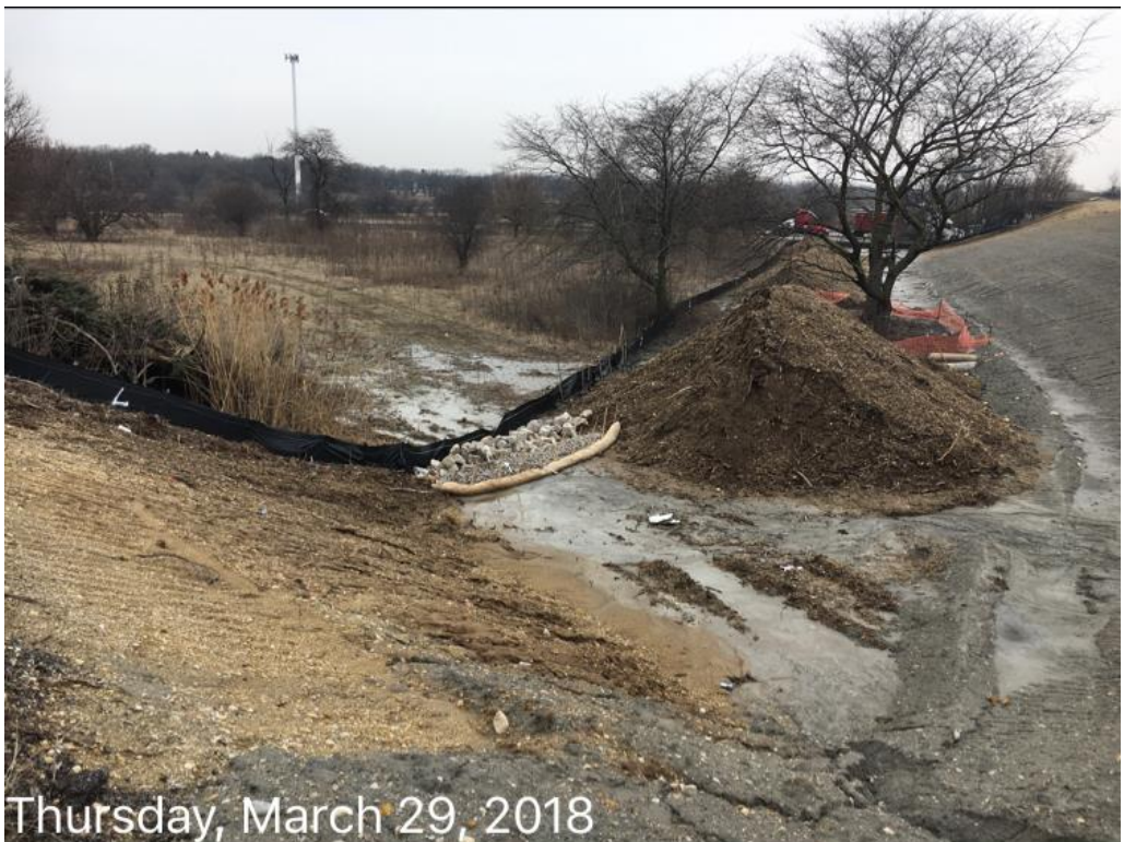
Figure 1: Sedimentation log, rock check dam and silt fence utilized to protect off-site drainage between I-55 and the I-55 northbound exit ramp, facing east.
