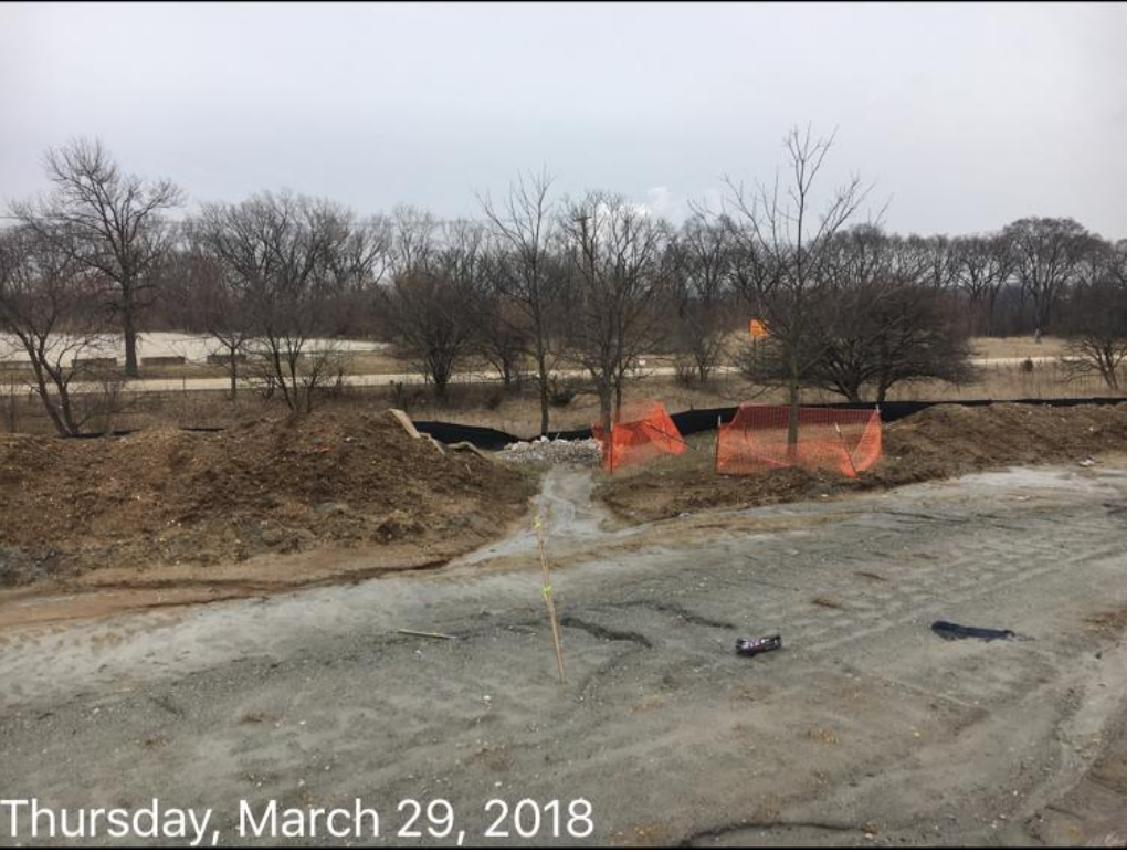
Figure 2: Sedimentation log, rock check dam and silt fence utilized to protect off-site drainage between the I-55 northbound exit ramp and Frontage Road, facing southeast.
