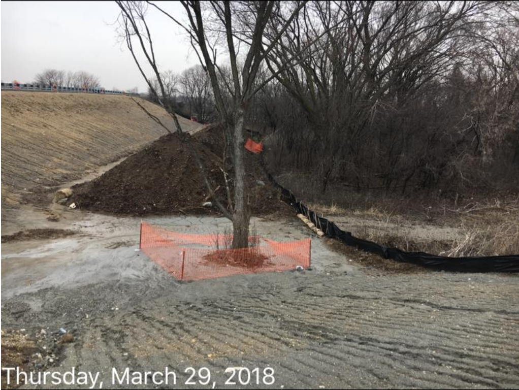
Figure 4: Silt fence and sedimentation log in good condition along east side of I-55, west of the northbound entrance ramp.
