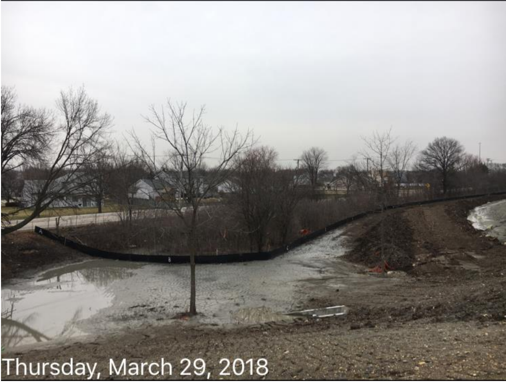
Figure 3: Silt fence in place between the southbound I-55 exit ramp and Frontage Road, facing north.
